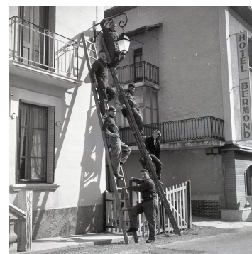
Installation éclairage public 1967
